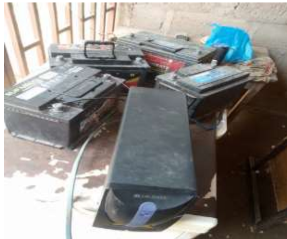
Figure 4. Four batteries connected in series
