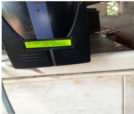
Figure 3: Four batteries in series
